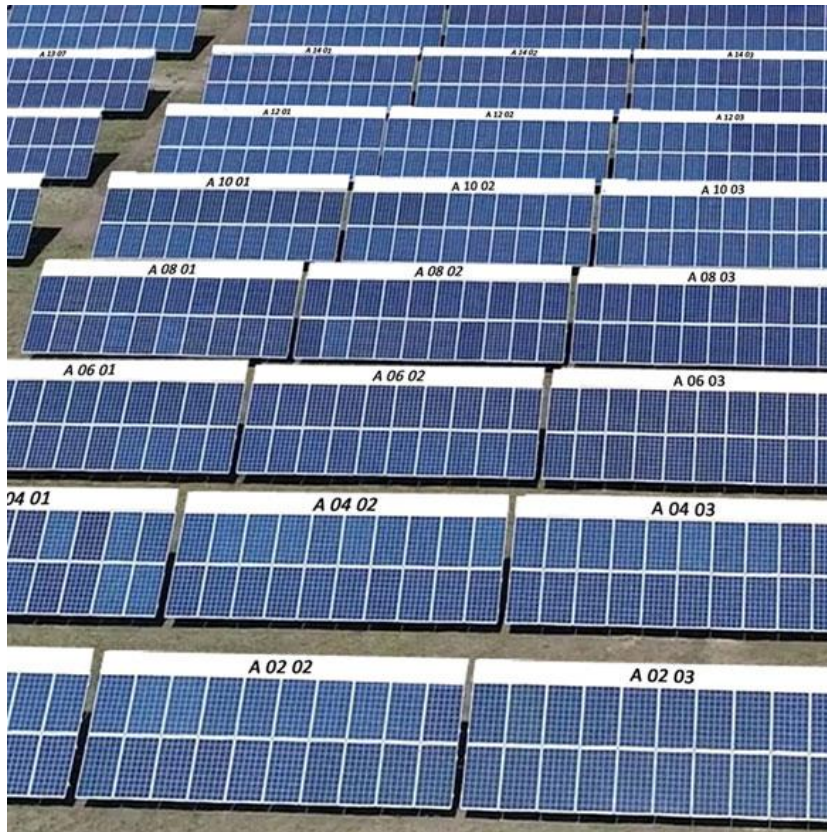
Figure 3.4 Solar panel identification labels
