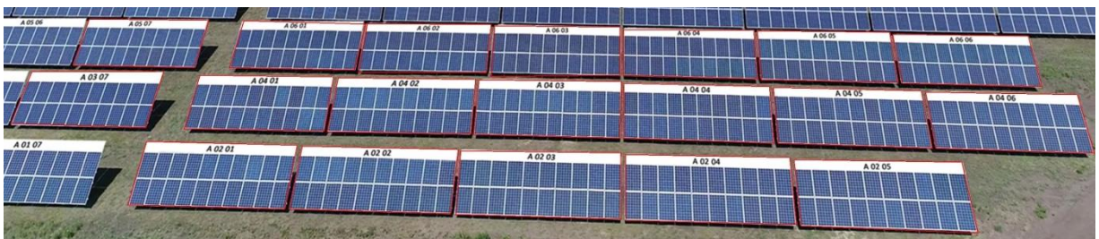
Figure 4.3 System screen - Solar panel identification
