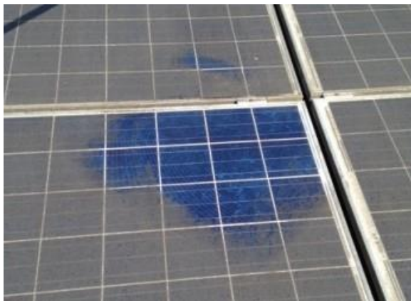
Figure 3.5 Solar panel cover with dust
