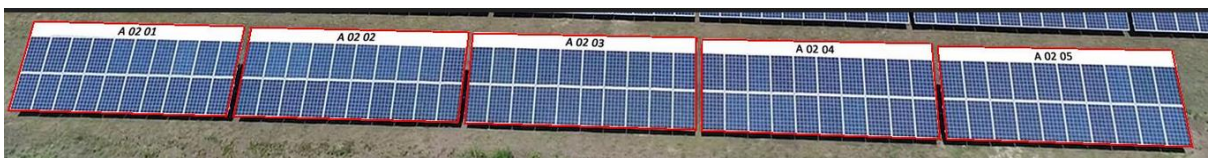
Figure 5.12 System screen - Solar panel identification
